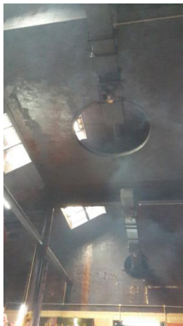
Figure 16. Extract ducts intrude in Main Prayer Hall. (Source: Author, 2017)
