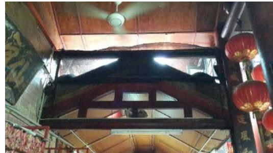
Figure 18. Surface mounted services. (Source: Author, 2017)
