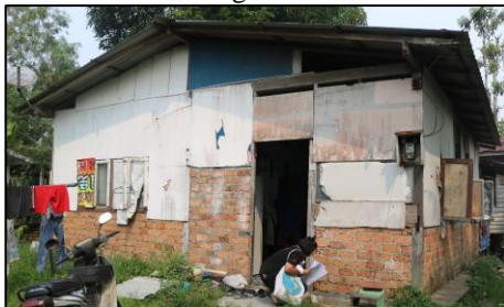
Broken external ceiling and leakages
