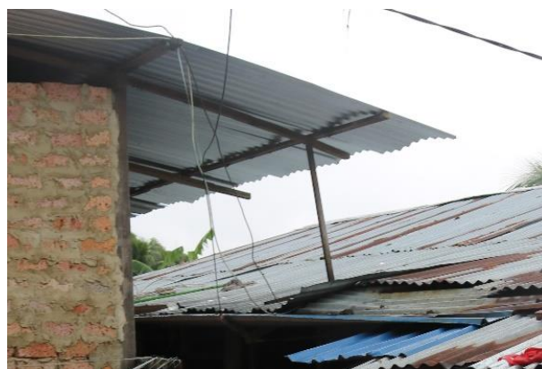
Figure 4: Roof of the new semi-detached house, which is lower than the main house
